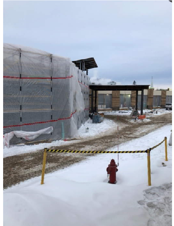
After scaffolding is installed on the exterior, it is enclosed as pictured. This is because the mortar must be installed in warmer temperatures in order to properly set.
