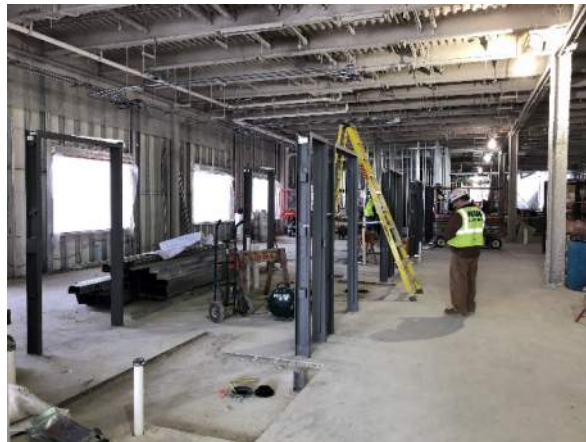
Stud walls and frames are being installed on the upper level of the new Clinic / Med Surge addition, MEP rough ins will follow.
