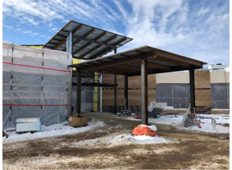
An exterior view on a blue sky day of the new canopy. Stud framing began for the new entrance.
