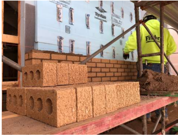
A Findorff Mason Foreman is installing brick on the exterior façade. This is a view from the other side of his work station.
